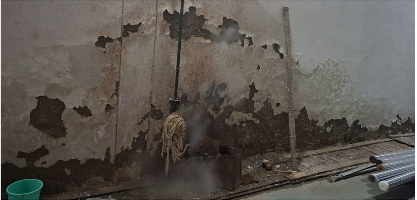
Image 7: Open Pipes Releasing Steam
