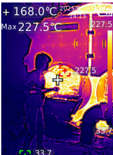
Image 14: Thermal Image of Boiler Unit
